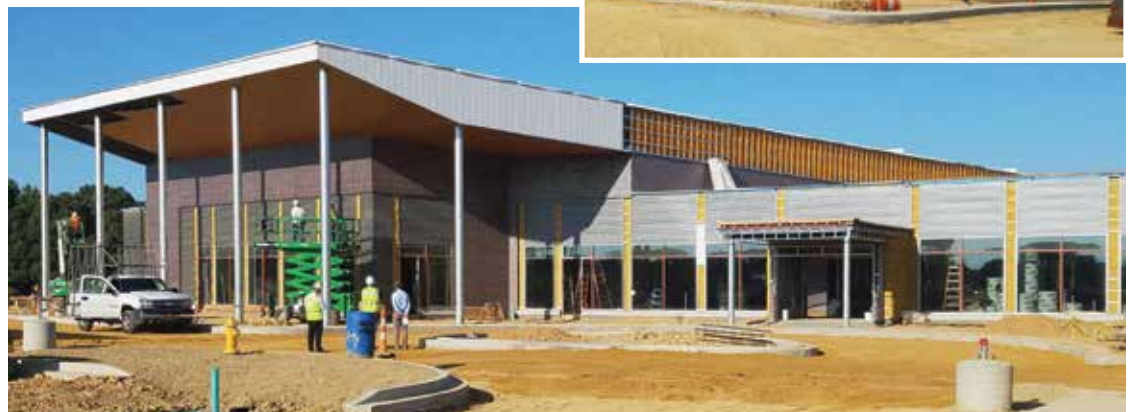
Construction of the Leonardtown Library and Garvey Senior Activity Center. Photos courtesy St. Mary's County Library.
